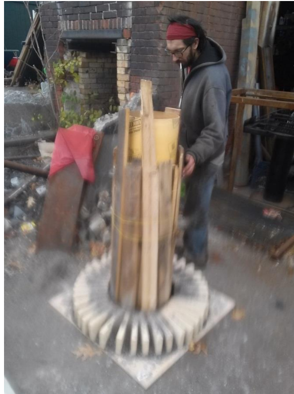
FIGURE 4. FURNACE STRUCTURAL SUPPORT TUBES.
