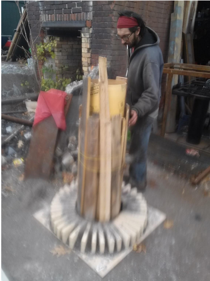
FIGURE 38 FURNACE STRUCTURAL SUPPORT TUBES.
